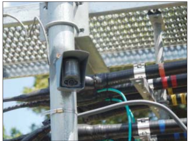
This camera gives a straight view from the cable tray looking outward, revealing any possible intruders to viewers at the security monitoring center. Metal thieves might be attracted by the copper in the wires shown here covered with green insulation.
