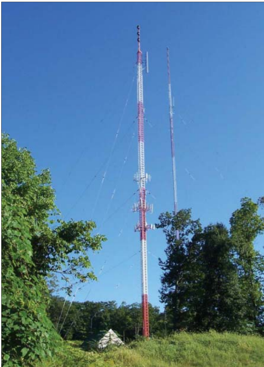
The newer, 367-foot tower, constructed in 2000, appears at the left of the tower built in 1990. The newer tower is designed to support its extension as high as 608 feet with a multi-ton load, so it has plenty of capacity for additional tenants including some that might want the highest possible antenna positions.
