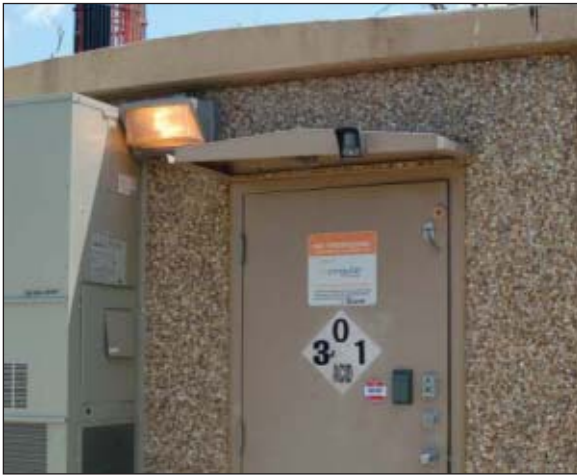
This view of a shelter shows the camera above the door and a proximity card reader on the door above the doorknob. The camera also views any approach to the air conditioner. Some thieves have removed air conditioners to gain entry to the building and have stolen all or part of the air conditioners for the metal they contain.
