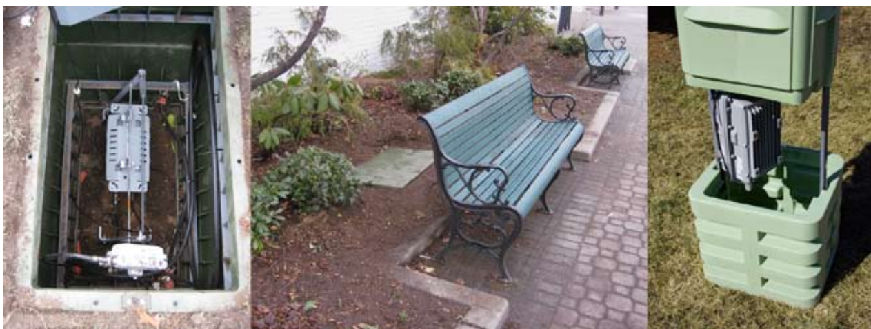
Figure 5. BelAir 100S vault and pedestal installations.
