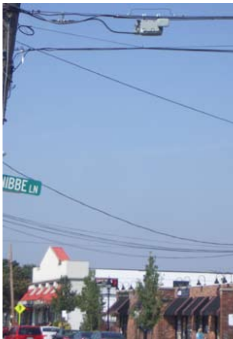
Figure 4. BelAir I00S deployed on aerial strand.
