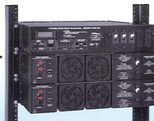
Site Power System
